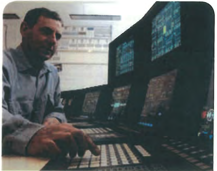
Advanced process control systems in the control room provide power station operators with the ability to see and manage the process and potential emissions.
