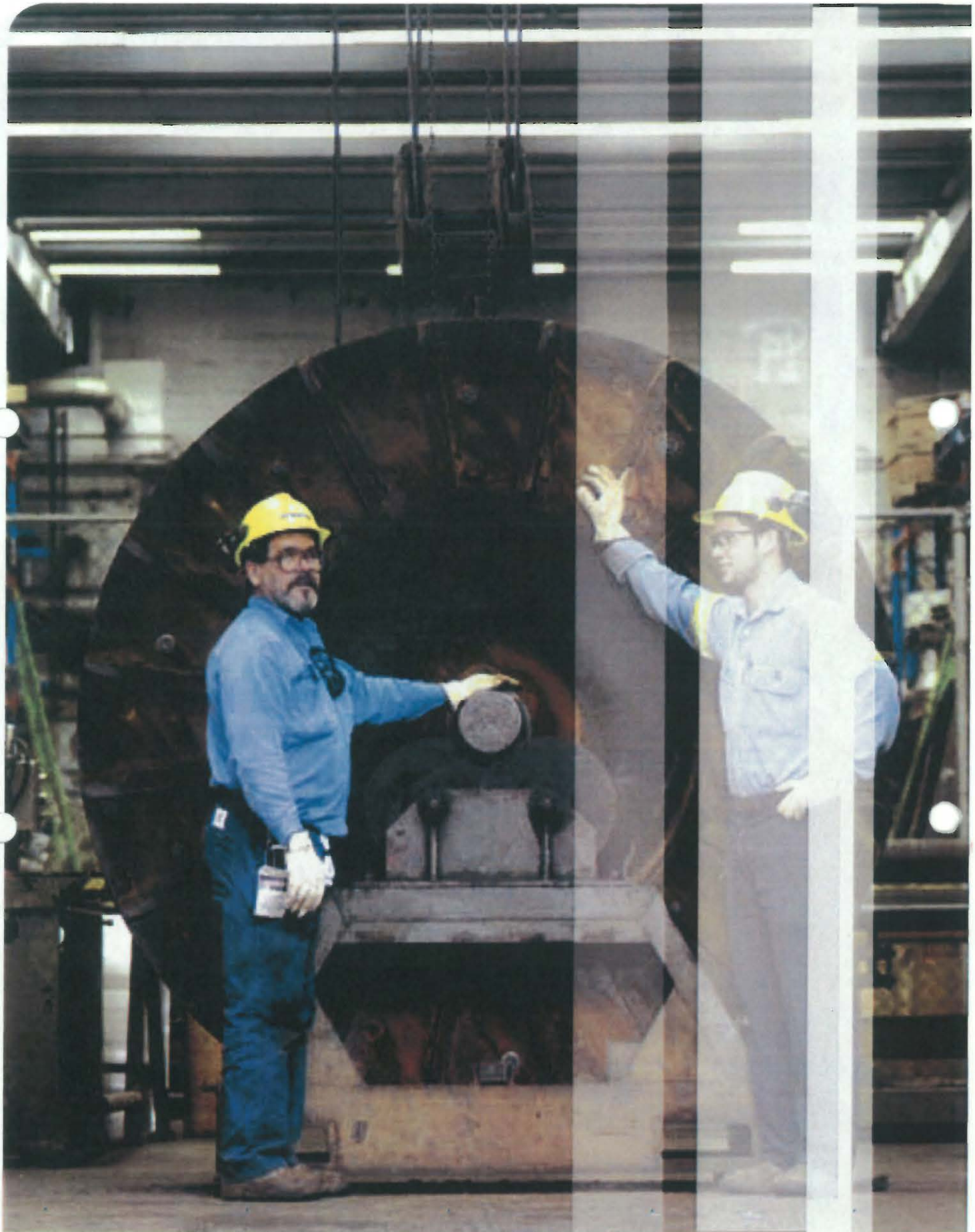
Pulveriser mill wheels crush the coal to a 'talcum-powder' consistency before it's air-blown into the boiler.
