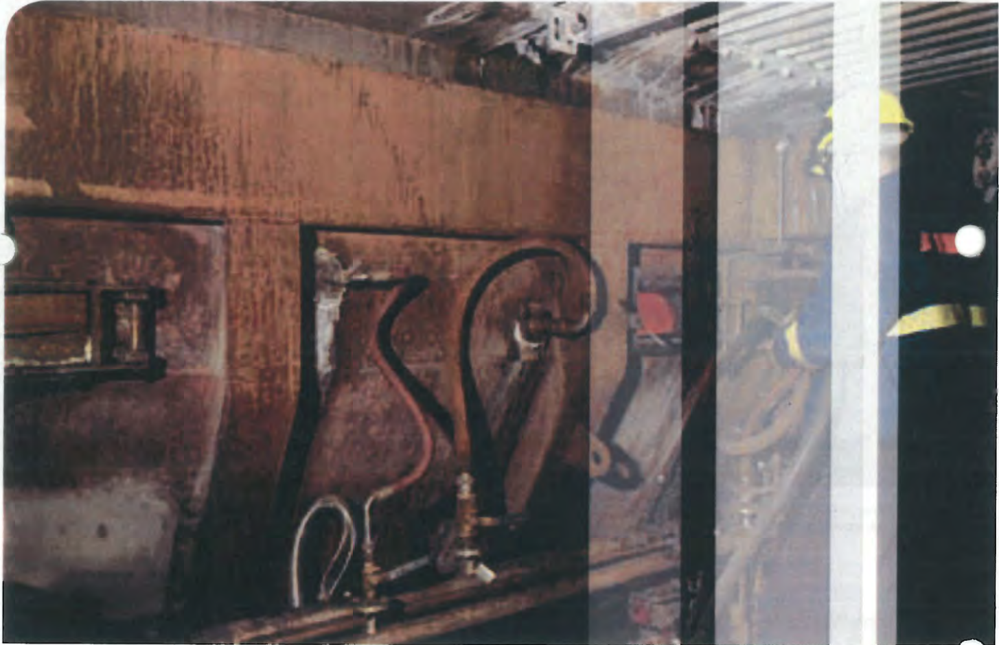
Fire prevention is one component of Anglesea power station's comprehensive crisis management plan.
