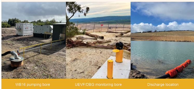
WB16 pumping bore
